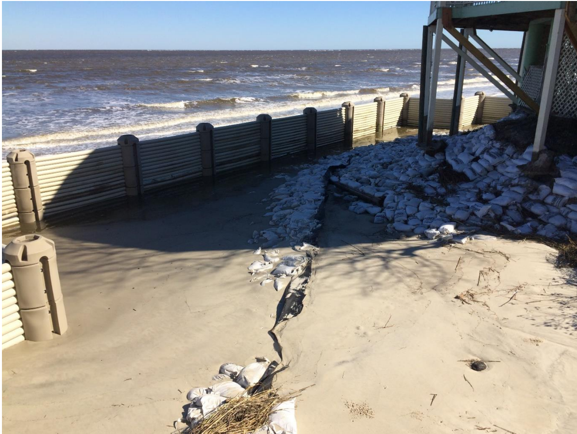
Figure 30. Typical trench issue on site (caused by scour as water exits the WDS and insufficient spacers; photo taken: 11/20/15).
