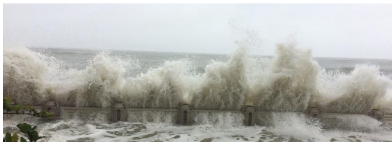
Figure 6. Breaking wave hitting area of WDS with only one line of resistance. Significant penetration is expected without controlled fill behind the WDS (see recommendations and conclusions section).
