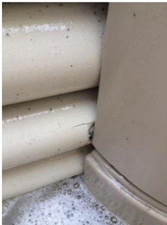
Figure 5. Cracked panel following direct wave hits associated with extreme tides.
