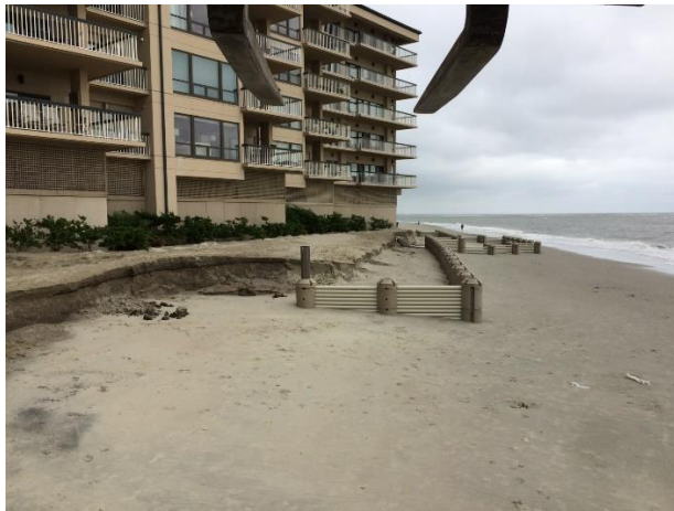
Figure 7. Advancing scarp adjacent to WDS and insufficient return of WDS (9/23/15). This figure shows how the WDS is intended to work where the scarp line behind the system is reduced relative to the adjacent property. Had the third tier as proposed been provided prior to this figure, the scarp line at the building corner would have been further from the building.
