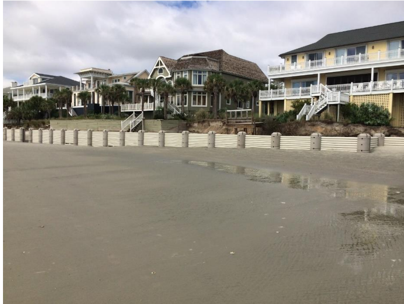
Figure 18. Wave Dissipation System at Beachwood East (10/11/15).
