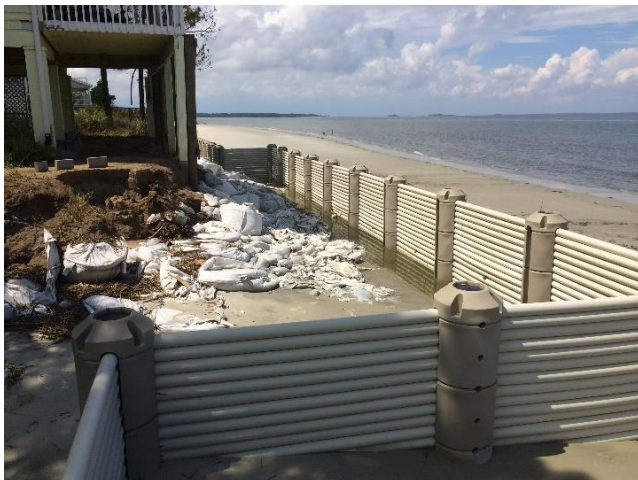
Figure 29. Typical temporary trench issue on site (caused by scour as water exists the WDS and insufficient spacers; photo taken: 9/8/15).
