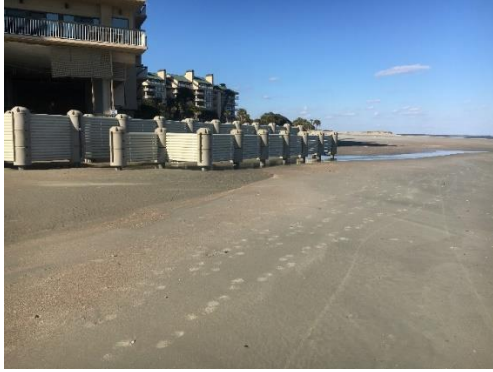
Figure 12. Severe beach lowering at OC prior to pile lowering (picture taken 2/25/16).
