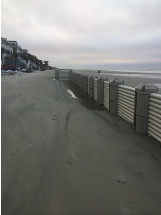
Figure 20. Typical trench at Beachwood East during the previous quarter report period (caused by scour as water exits the WDS; photo taken: 11/4/15).
