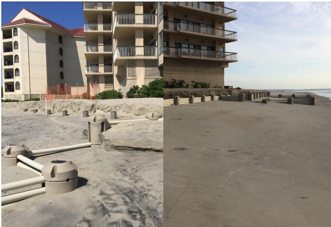
Figure 2. Wave Dissipation System prior to (8/14/15) and after (9/3/15) installation of horizontal panels in area where piles were not covered with housing units during initial construction. Note exposed piles following erosion event on left.
