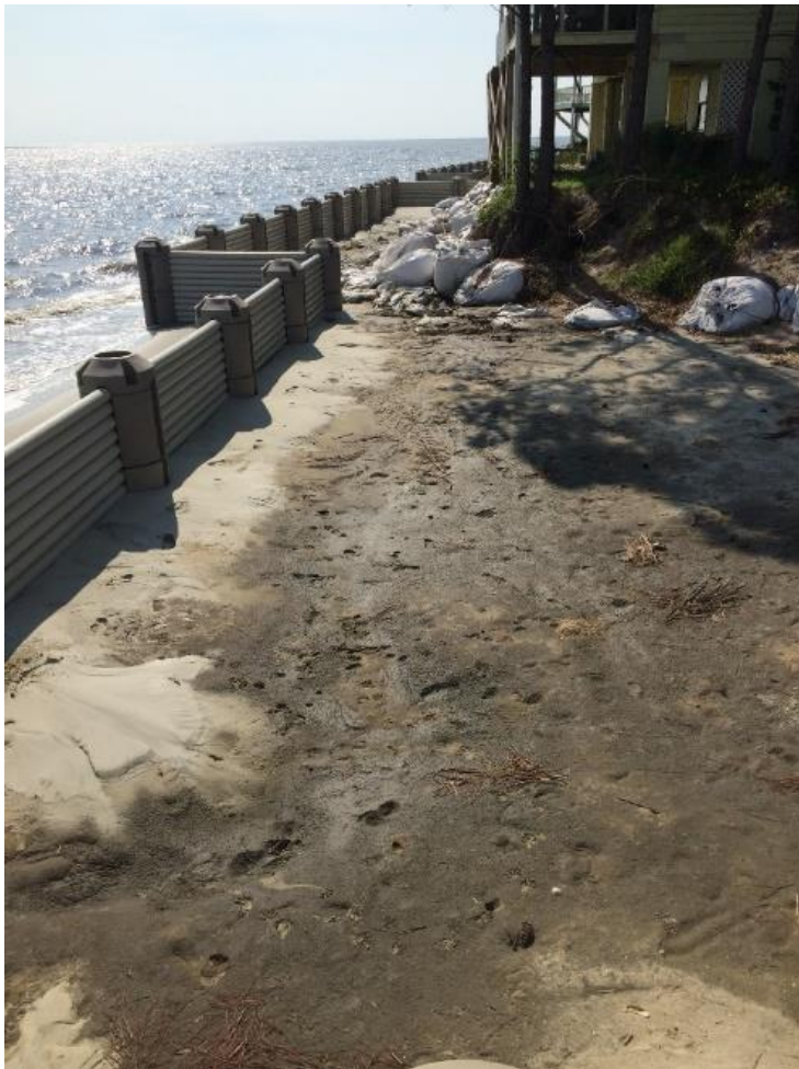
Figure 27. Initial, very localized, accretion (typical with no spacers) behind WDS (photo taken: 7/17/15).
